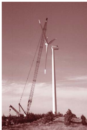
Our purchase of wind energy credits helped finance the construction of the first large-scale Native American-owned wind turbine. This wind turbine, located on the land of the Rosebud Sioux Tribe in South Dakota, was dedicated in May 2003.
